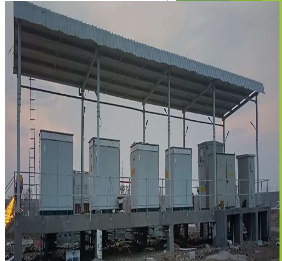
Solar Inverter PEB Structure Shed
